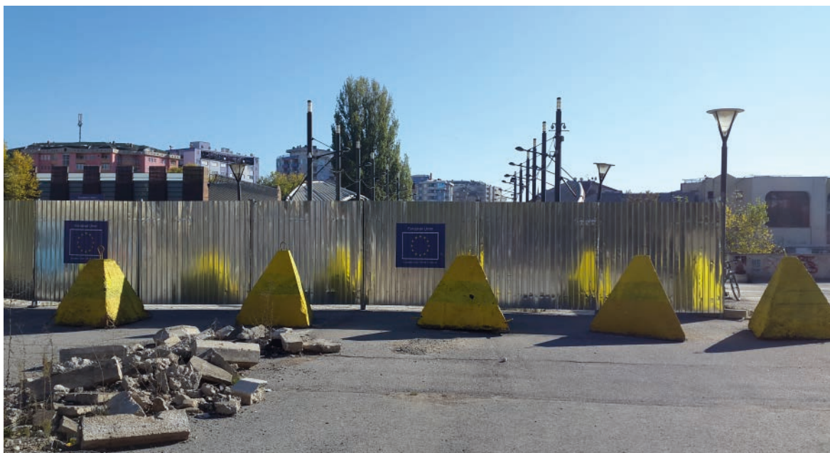
View of the works on the Ibar/Ibri bridge from North Mitrovicë/Kosovska Mitrovica
